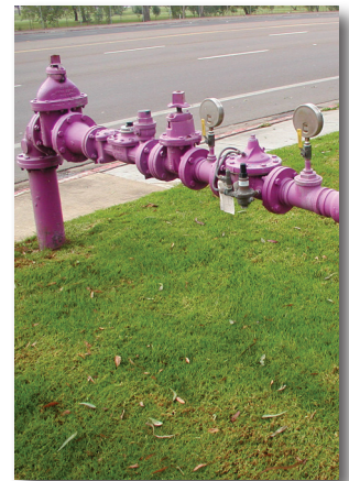
Distinctive purple pipes identify recycled water systems.
