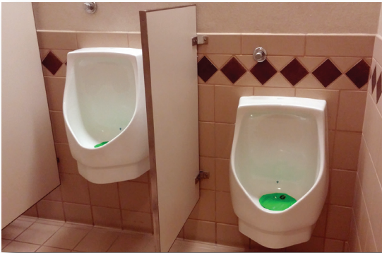
Nine waterless urinals installed in the Water Authority's headquarters can each save approximately 26,000 gallons per year.
