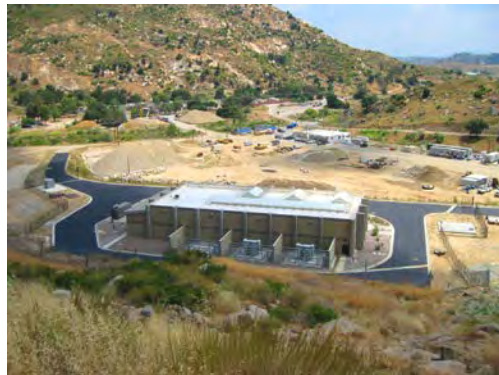
The San Vicente Pump Station will be utilized to supply untreated water during emergency events.
