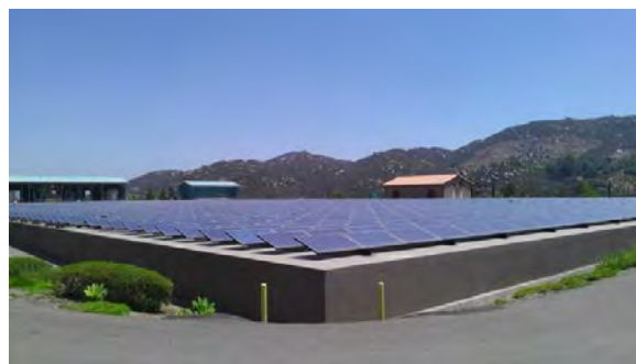
The Water Authority has identified various solar opportunities to supplement its renewable energy portfolio, similar to the solar panels installed at the Twin Oaks Valley WTP.
