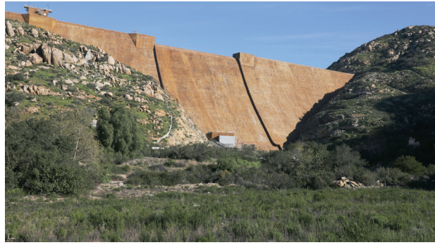
The San Vicente Dam Raise, completed in 2014, more than doubled the reservoir's capacity.
