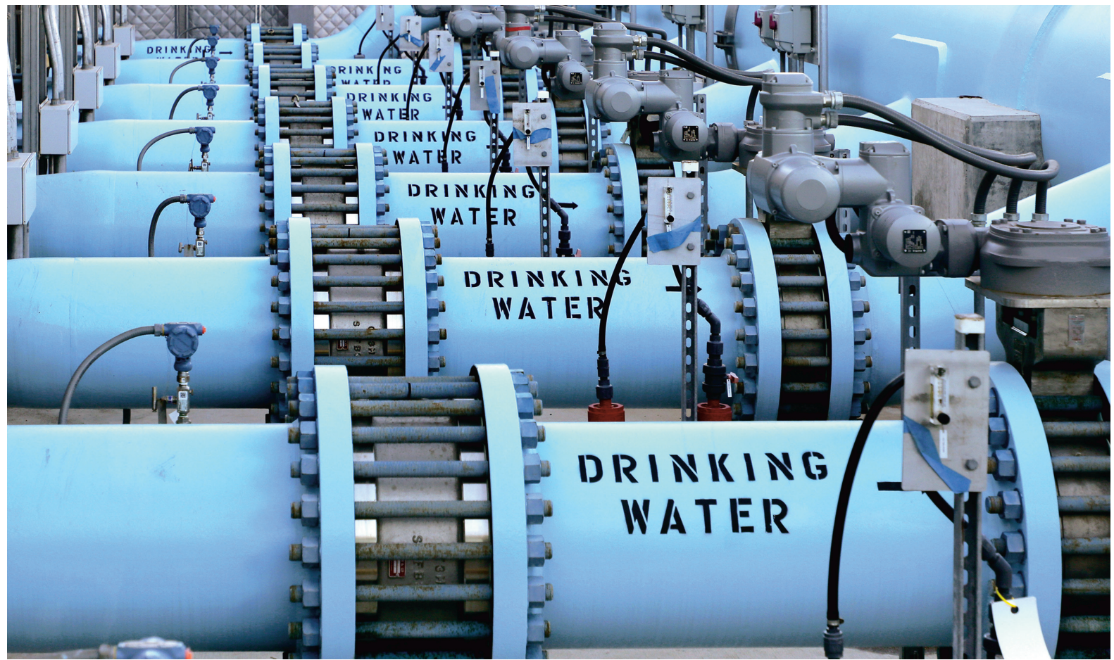
The Claude "Bud" Lewis Carlsbad Desalination Plant produces 50 million gallons a day of desalinated seawater. Completed in 2015, the plant provides the region with a highly reliable, drought-proof water supply that meets about 10 percent of regional demand.
